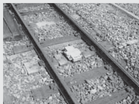
Automatic train stop (ATS) device
